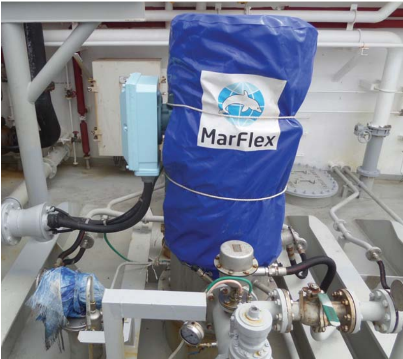
Marflex Variable Frequency Drive Cargo pump.
